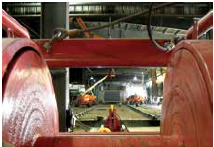
A large winch was mounted to the mill floor to roll the 1 million pound dryer into place. A second installation using this method is now underway in the Southern U.S.
