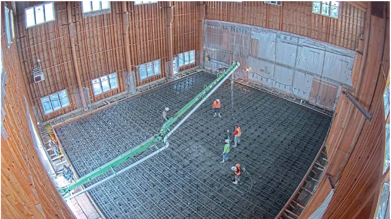
The “strong floor” in the APA lab’s new addition will allow for the testing of taller and heavier assemblies.
