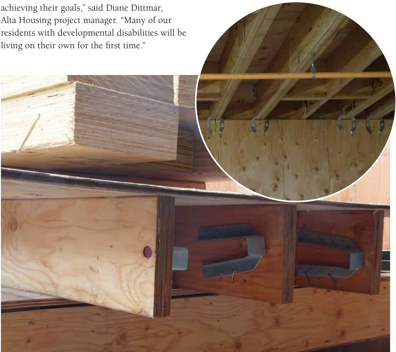
Prefabricated floor cassettes and laminated veneer lumber were used as a cost-effective solution throughout the structure.
