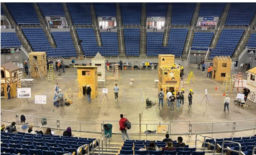
Construction underway at the Lawlor Event Center at the University of Nevada Reno, for the American Society of Civil Engineers (ASCE) Study Symposia 2023 Timber-Strong Design Build Competition.
