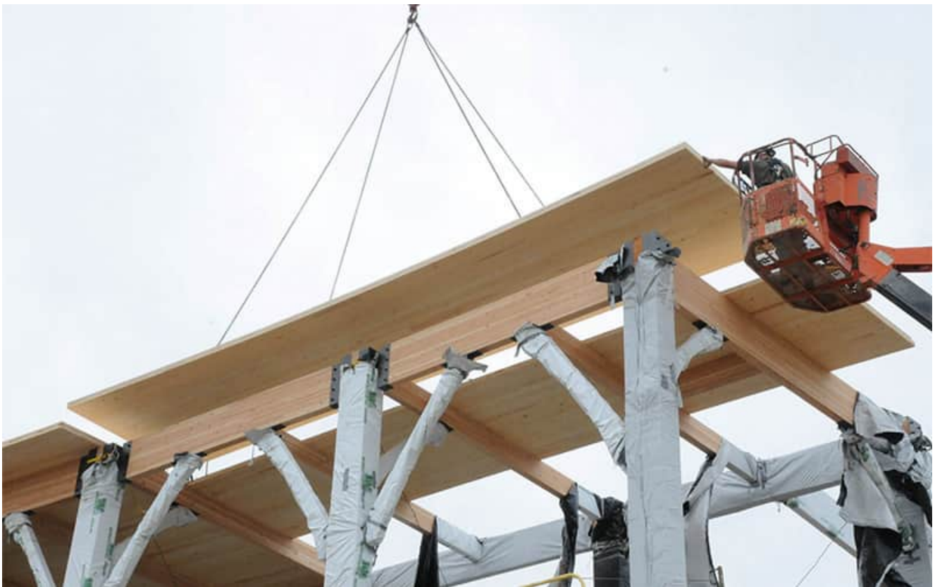
Engineered wood products and mass timber can be ordered in custom and longer lengths and even pre-cut framing packages, all of which help reduce construction waste.
